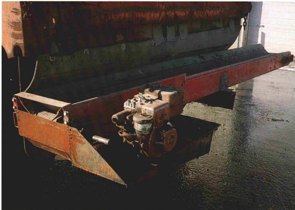
View of truck-mounted conveyor-belt device used to deliver crushed stone to drainage trenches.
