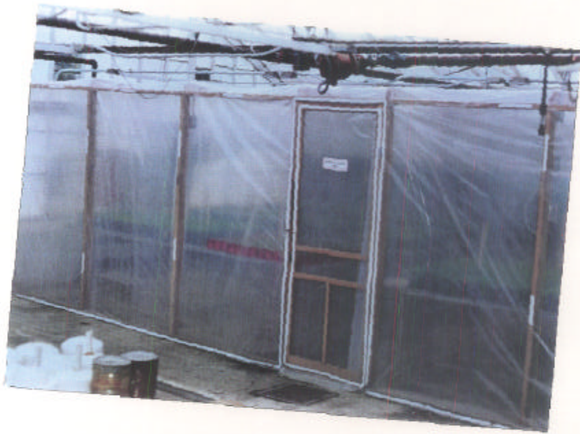
Figure 2. Inside the greenhouse bay a 27' x 16' x 8' wooden frame was built. Two layers of greenhouse polyethylene covers the structure. Air is forced between the double layer of plastic to create a layer of insulation.
